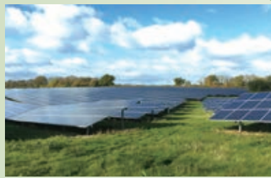
Picture of One of the UK Power Plants
